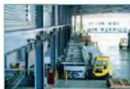
Logistics Conveyor System
